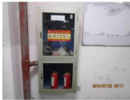
Fire extinguishers and hydrant
