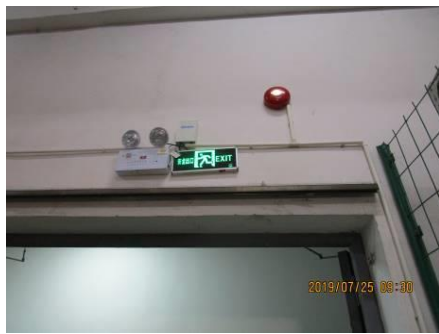
Exit, emergency light, fire alarm
