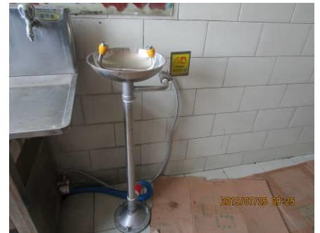
Eye washing facility
